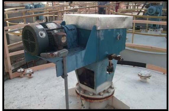
Reichhold created a metal "hat" to prevent water from entering their gearboxes.
