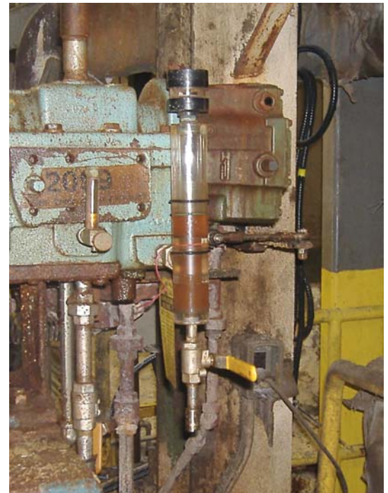
An Esco Oil Sight Glass & Level Monitor installed on a steam turbine at the Cargill Salt facility, St. Clair
