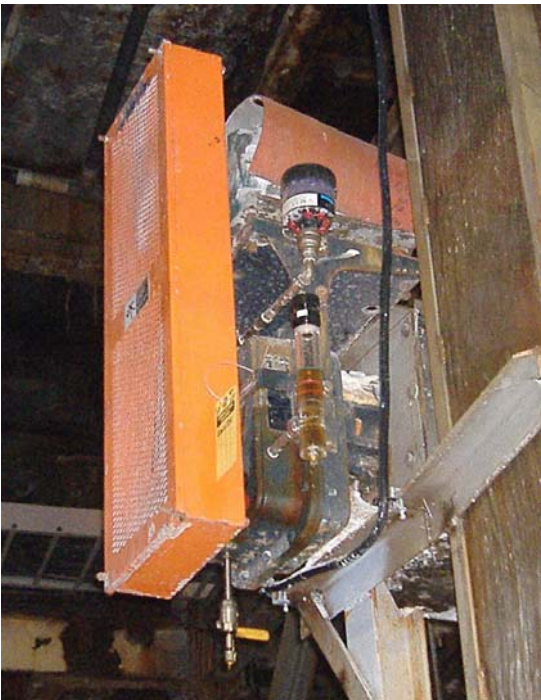
Great visibility from the floor: an Oil Sight Glass & Level Monitor installed 15' above the viewer.
